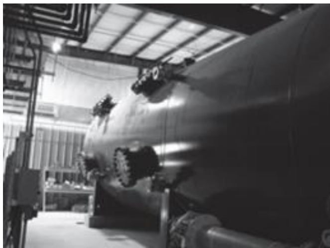
Figure 15.2 - Biological Activated Carbon Absorber (S. Hanson photo file)
